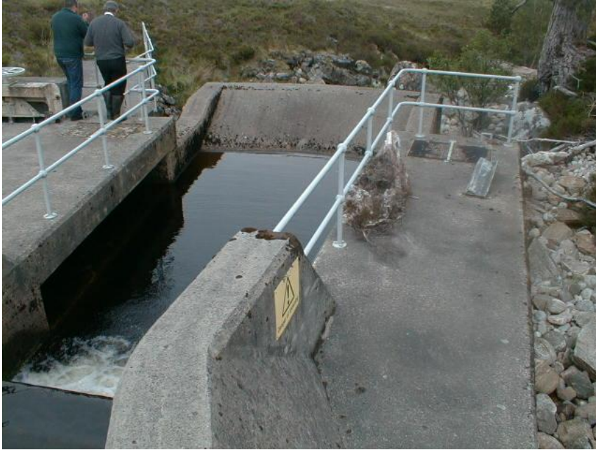
Picture 1: Scoop intake showing 'scoop' shaped central channel with side intakes. In high flow conditions the water continues over the crest of the intake and effectively scours the intake on every spill (photograph courtesy of Scottish & Southern Energy).
